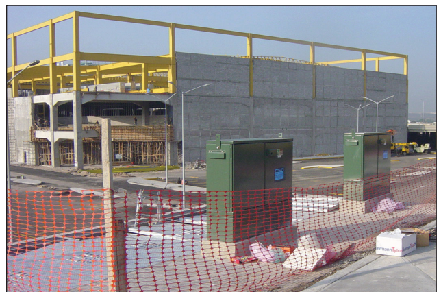
Photo 2. Low-voltage enclosure shown, with Vista units located in an underground vault.
