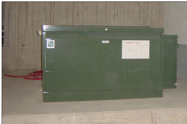
Photo 1. Vista unit located inside an electrical room.
